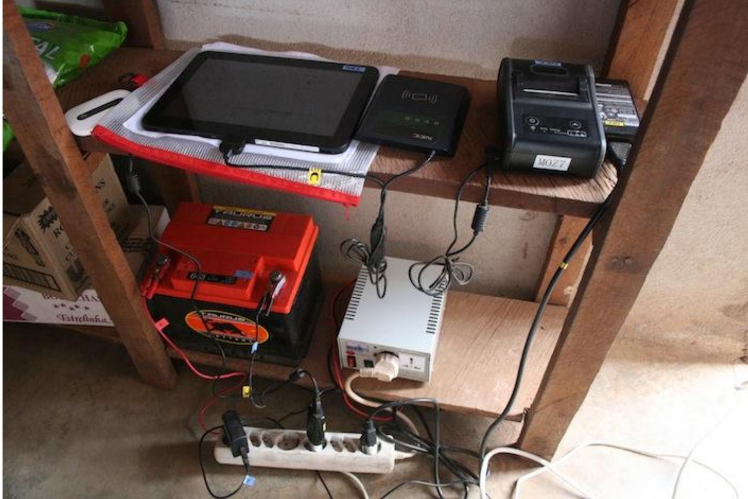
Equipment charged by solar panel
